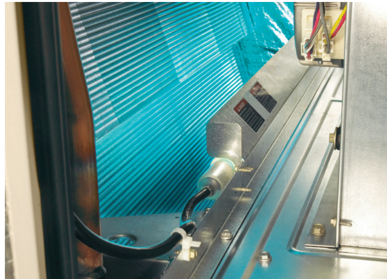
Example of UVC kit installed on Emperence rooftop unit
